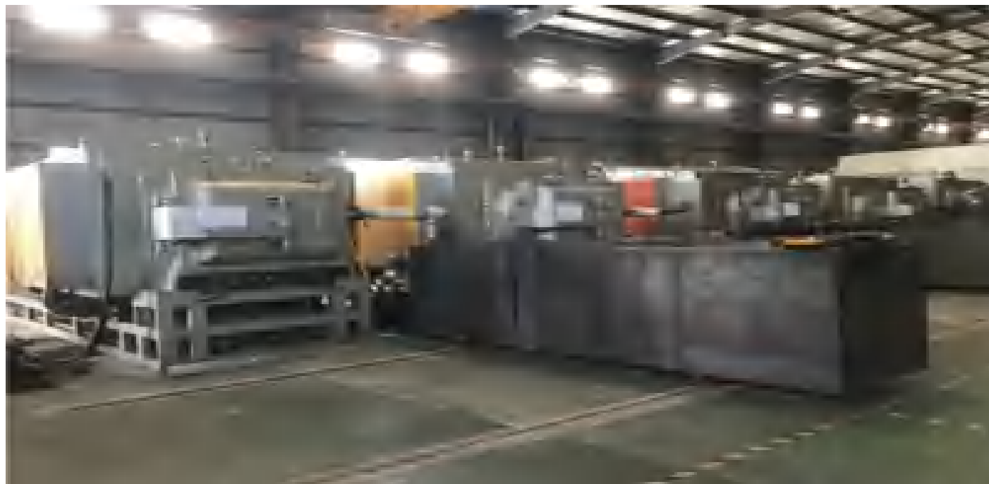
Fully Automatic Ultra-Microcrystalline Core Heat Treatment Production Lines (5 Lines)
